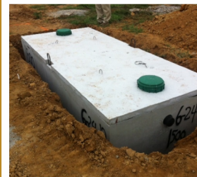
COMMON SEPTIC TANK
