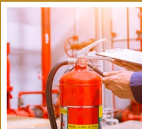
FIRE FIGHTING SYSTEM IN CLUB HOUSE
